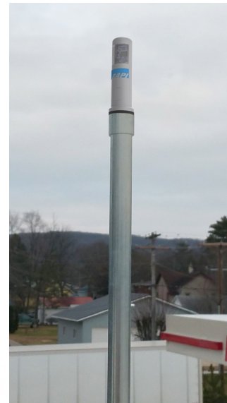
Sensor mounted in a parking lot facing north
